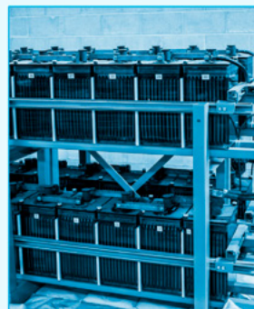
VRLA and Lithium-Type Batteries
